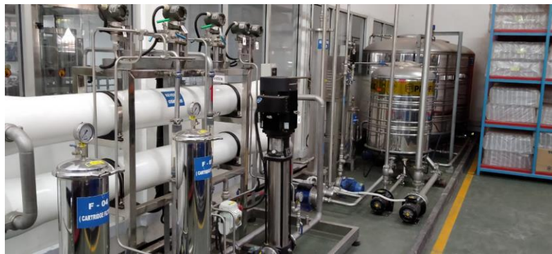
Gambar 1. Water Treatment Plan PUTOI PNJ (Sumber: Dokumentasi Pribadi)
